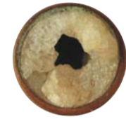
Cross section of a scaled hot water pipe.
